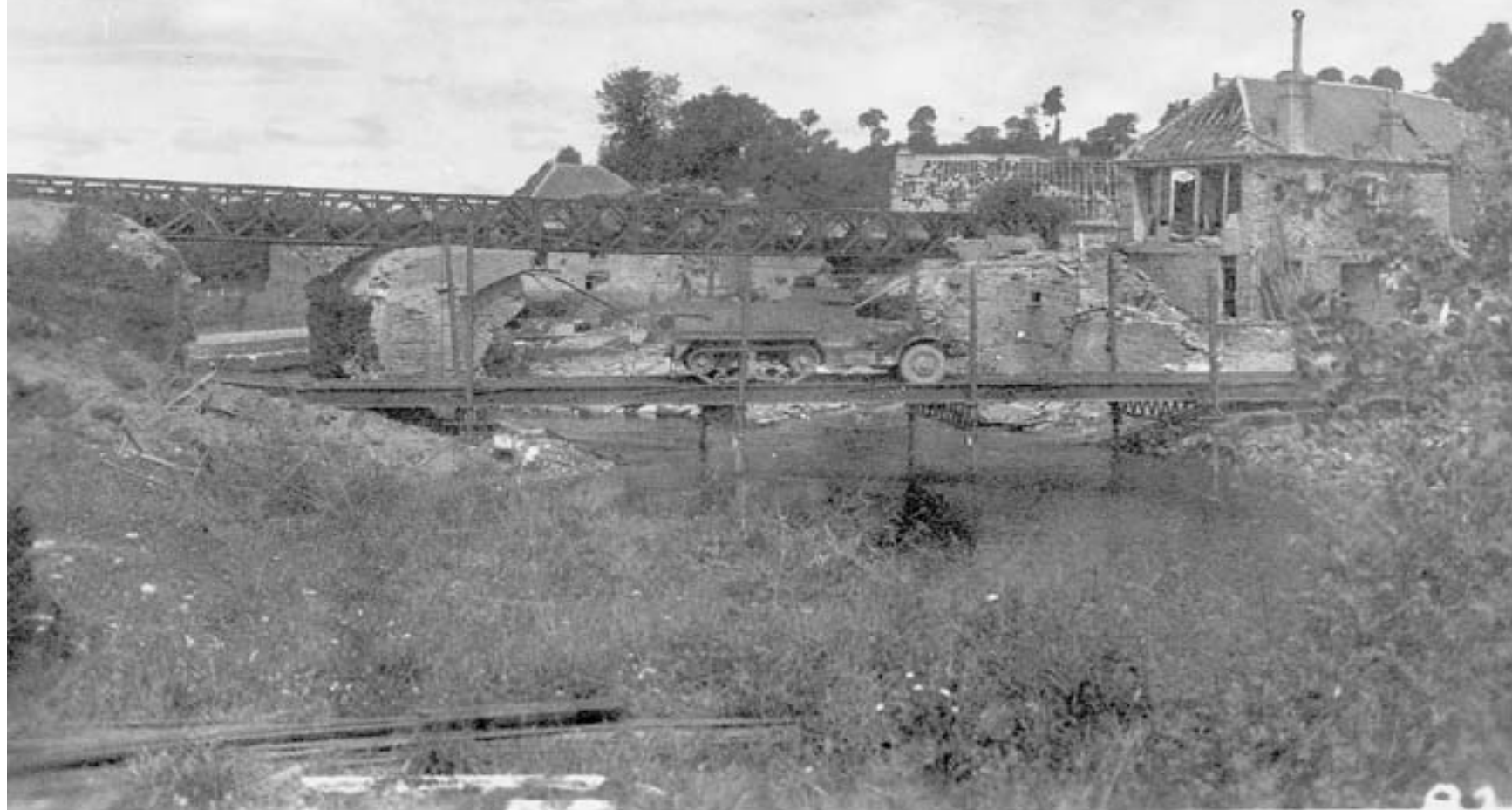
8232-8248 Including views of 110' TS-BB, 84' trestle tdwy. br. constr. by A Co., B Co., 82 Engrs. Candol, Normandy France. 28 July '44
