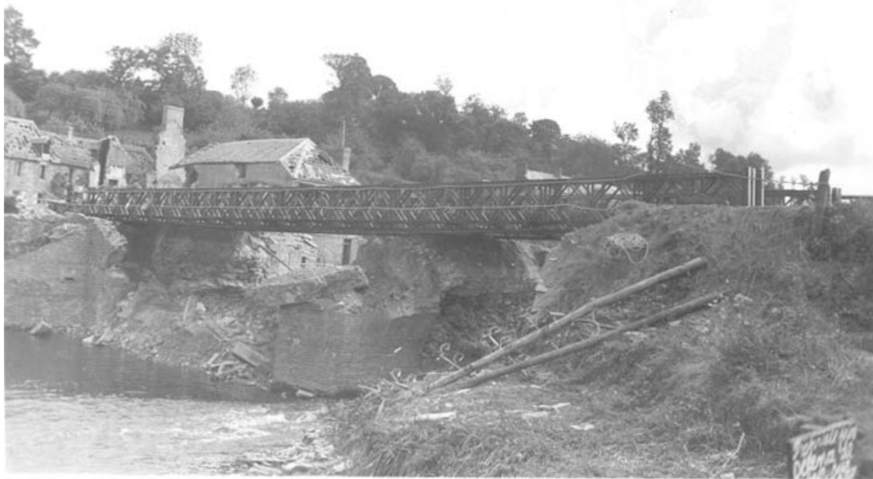
8232-8248 Including views of 110' TS-BB, 84' trestle tdwy. br. constr. by A Co., B Co., 82 Engrs. Candol, Normandy France. 28 July '44
