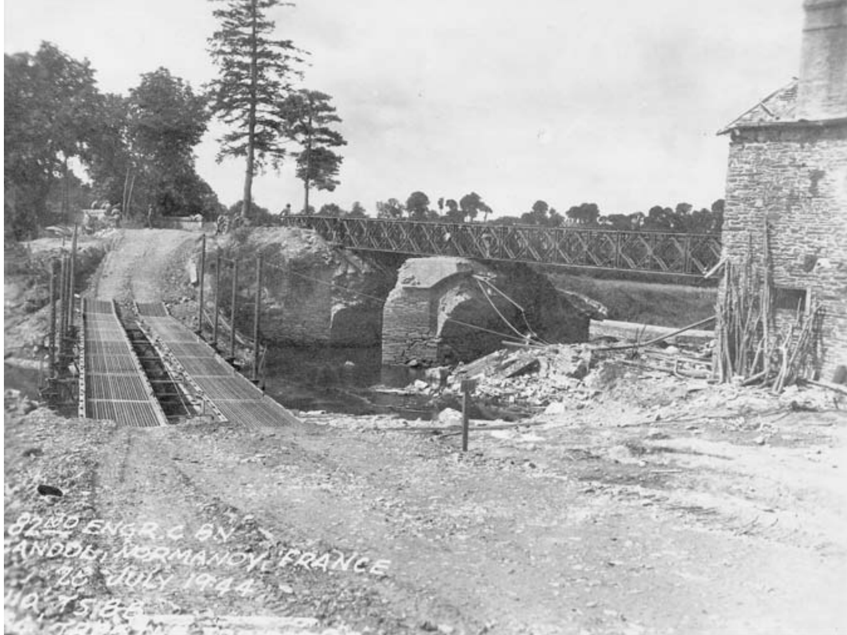
8232-8248 Including views of 110' TS-BB, 84' trestle tdwy. br. constr. by A Co., B Co., 82 Engrs. Candol, Normandy France. 28 July '44
