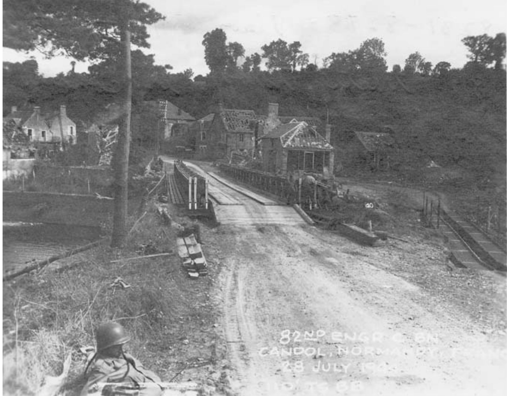
8232-8248 Including views of 110' TS-BR 84' trestle tdwy br constr by A Co. B Co
